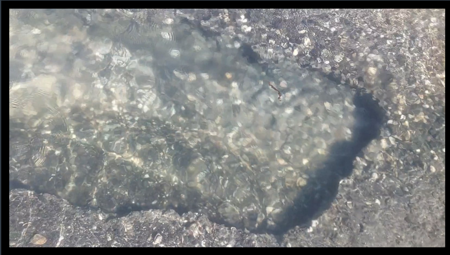
Footage showing the exit point of the leak, into the estuary
