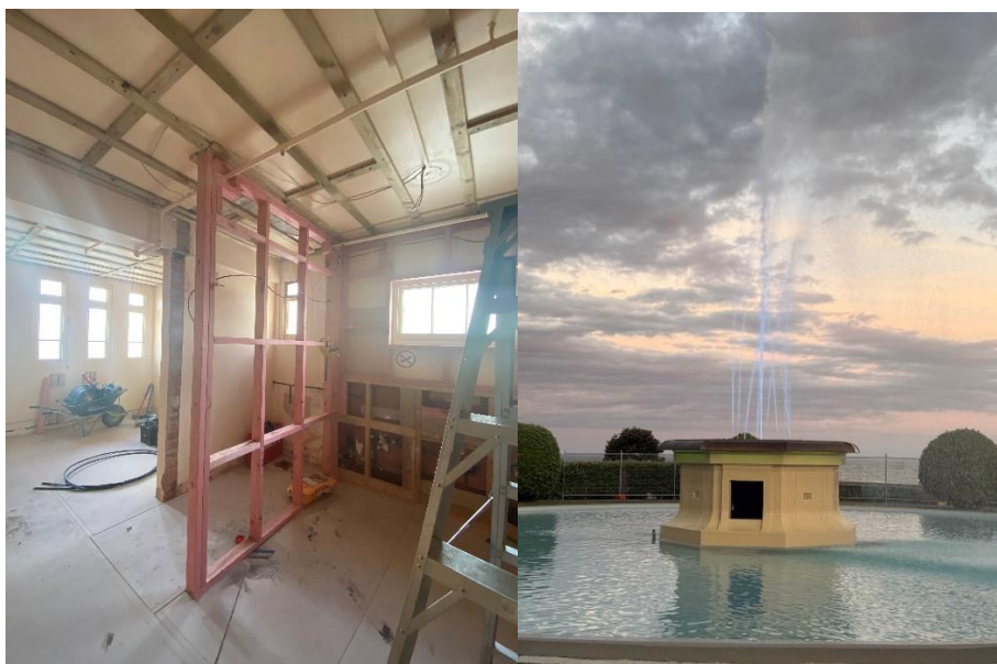
Photos above showing completed works at Tom Parker Fountain and works in progress at Municipal Theatre.
